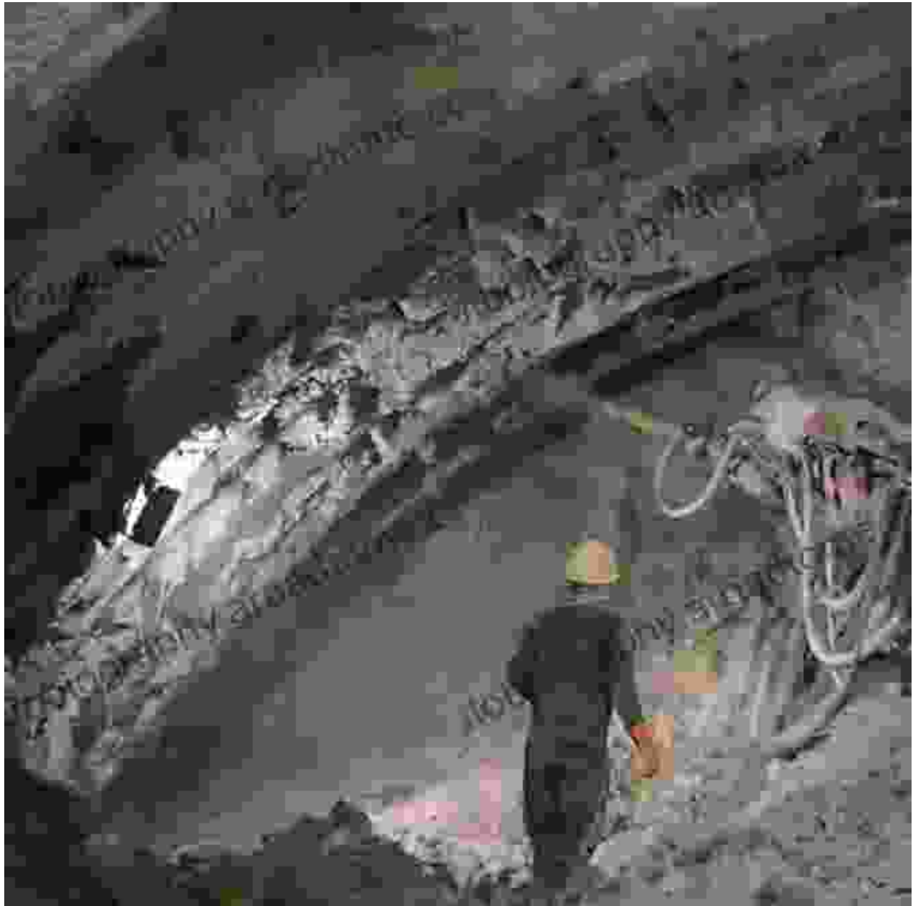
Rockbolts securing a tunnel to prevent rockfall and maintain stability.
